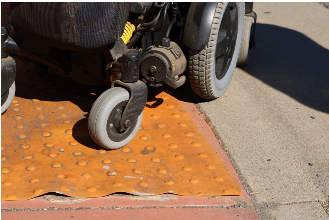
TRUNCATED DOMES AT CURB RAMP IN DISREPAIR.
