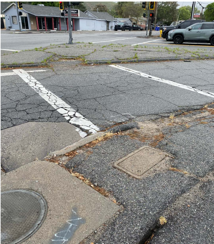
ABOVE: Cracked, uneven pavement and sidewalk at the West 40th Street / North Electric Avenue.
