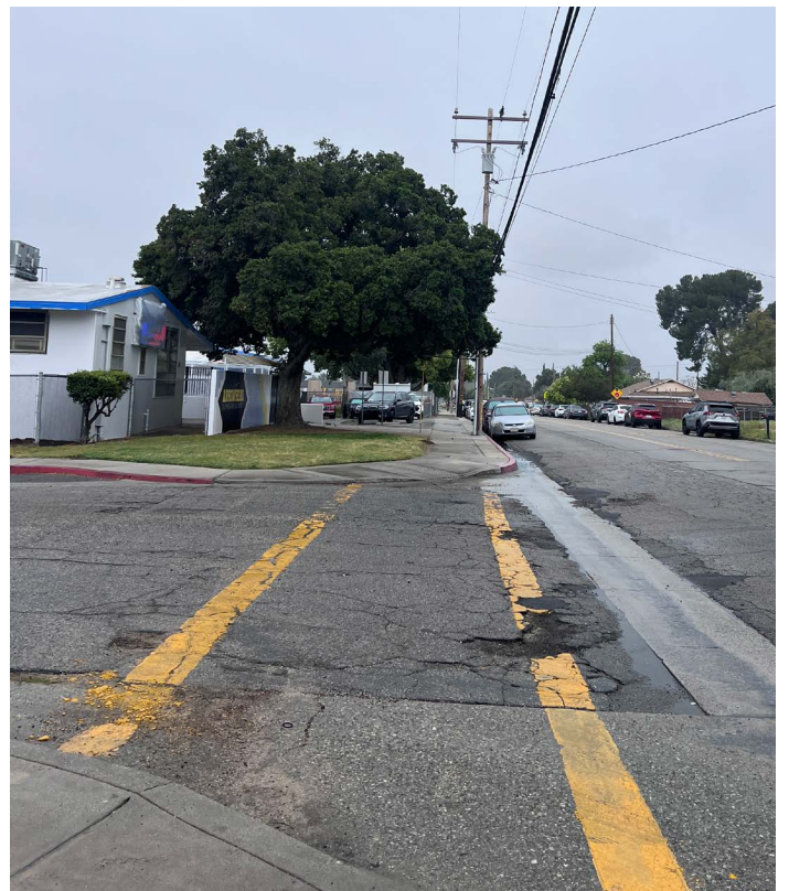
ABOVE: The pavement along Arrowhead Elementary School's campus is damaged.
