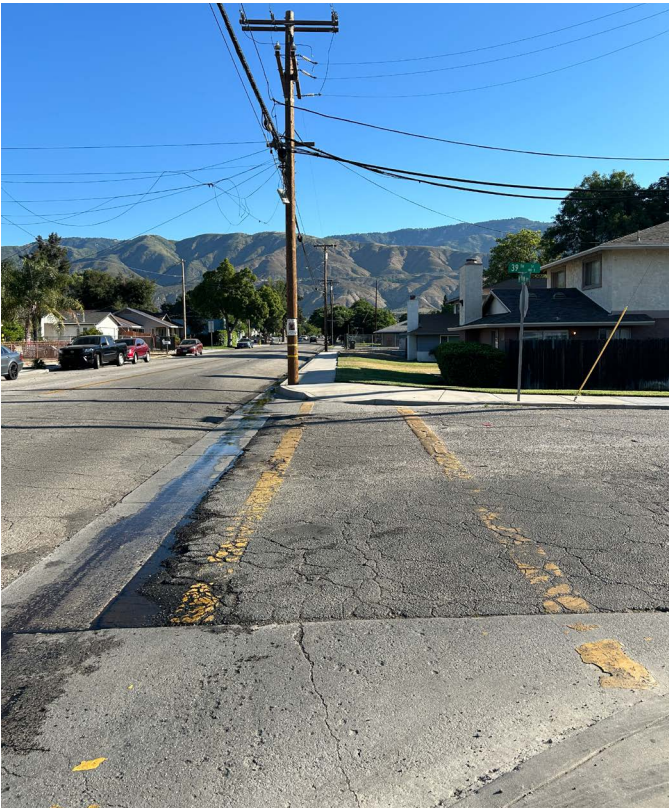
ABOVE: The crosswalk at North Mountain View / 39th Street is faded, and cracked, with potholes that collect water, which make it difficult for those traveling to and from Arrowhead Elementary School.
