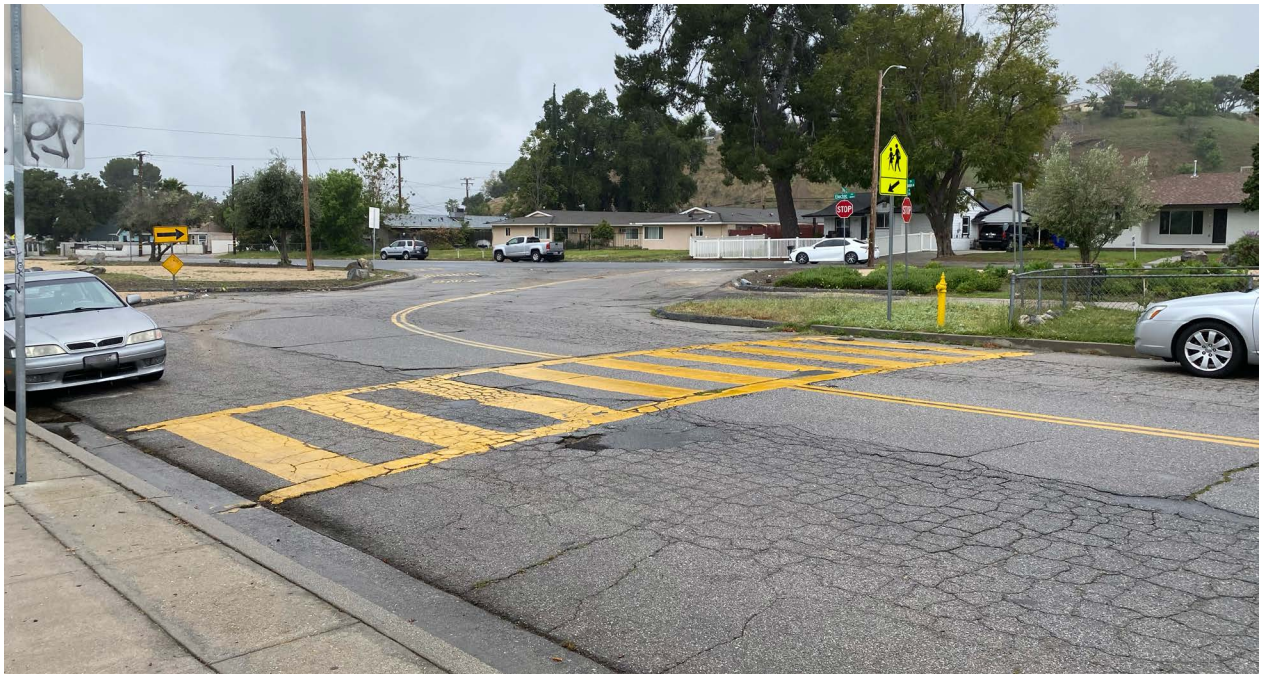
ABOVE: The North Electric Avenue / North Mountain View Avenue / North Palm Drive intersection poses many risks for those walking, biking, or rolling.
