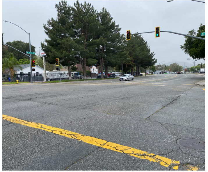
ABOVE: The North Mountain View Avenue / West 40th Street intersection is wide and difficult to cross safely in one pedestrian interval for some.
