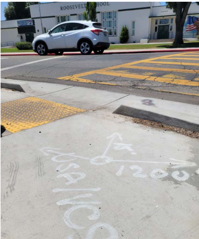
ABOVE: The curb on 10th Avenue across the street from Roosevelt Elementary is a tripping hazard when larger groups cross at the same time.
