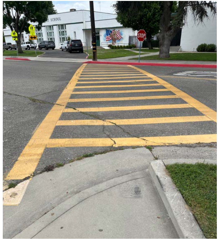
ABOVE: A curb ramp is missing on 10th Avenue in front of Roosevelt Elementary, forcing people to use the adjacent driveway.
