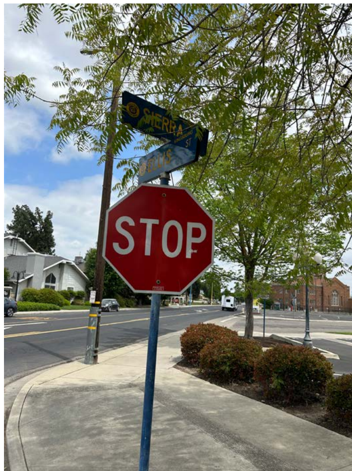
ABOVE: Obstructed view of Right Turn Only sign on the southside of Sierra Street (SR-201) and west corner of Washington Street.
