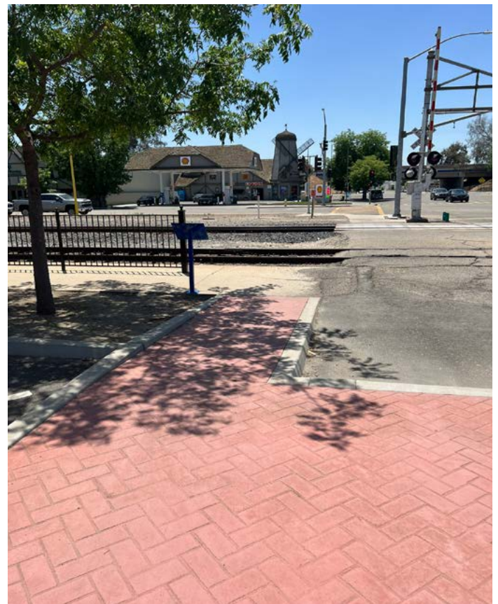
ABOVE: The curb ramp from Draper Street leads directly to the train tracks with no detectable warnings to alert people that they are entering a train crossing.
