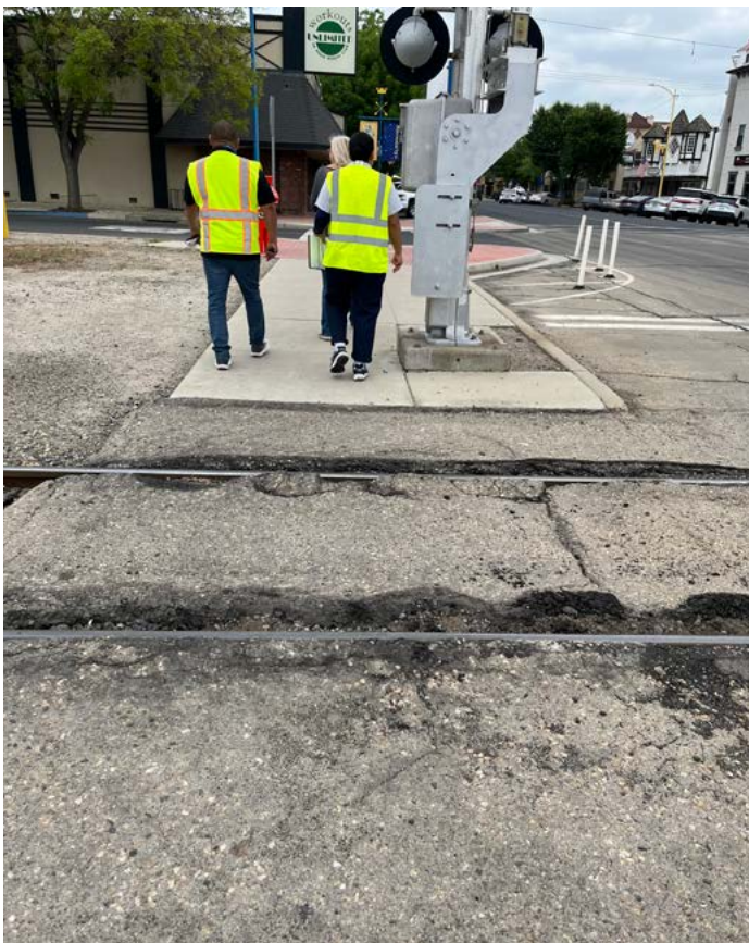
ABOVE: The pavement around the railroad track is in disrepair and poses tripping hazards.
