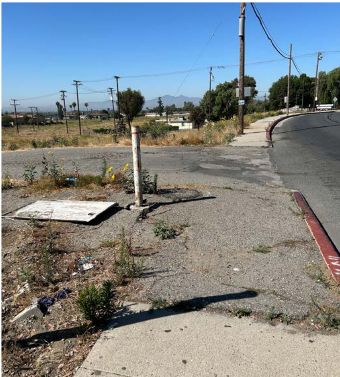
ABOVE: A cracked sidewalk on Riverview Drive connects to a dirt road that serves as a path to a small shopping center.
