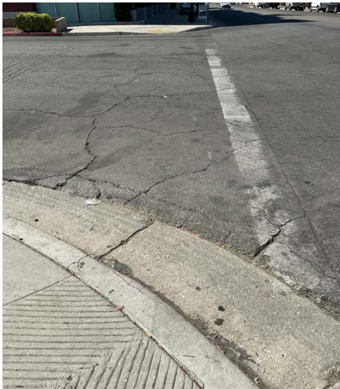
ABOVE: The crossing markings at the Baker Street/Lake Street intersection are faded and the road is cracked.
