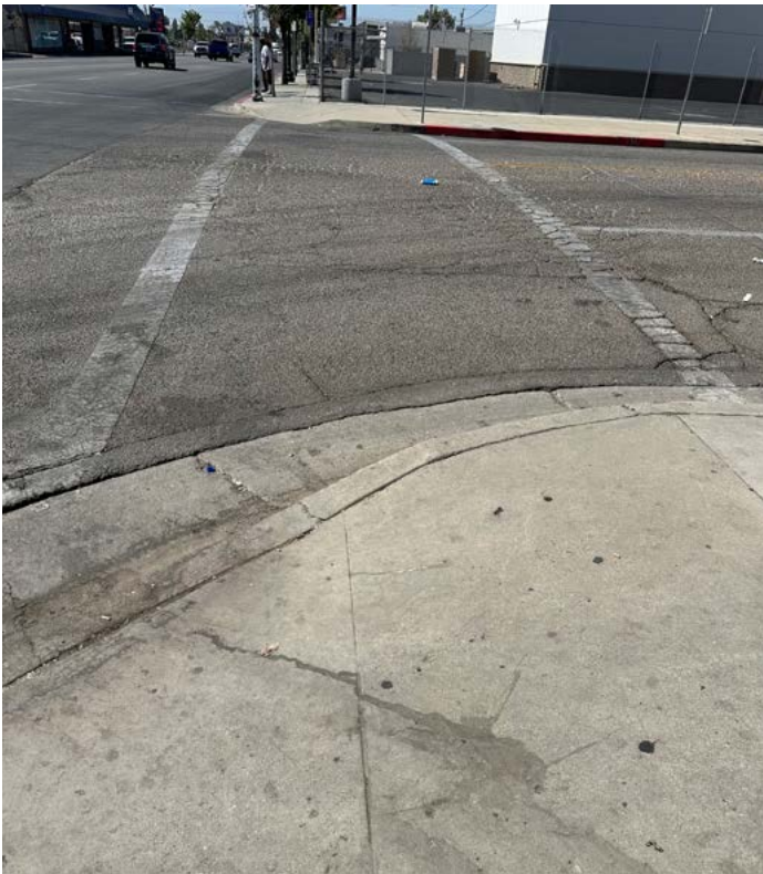
ABOVE: The crosswalk at the 21st Street/Baker Street intersection has faded paint and cracked street pavement, so drivers may be less aware of its presence due to its limited visibility.
