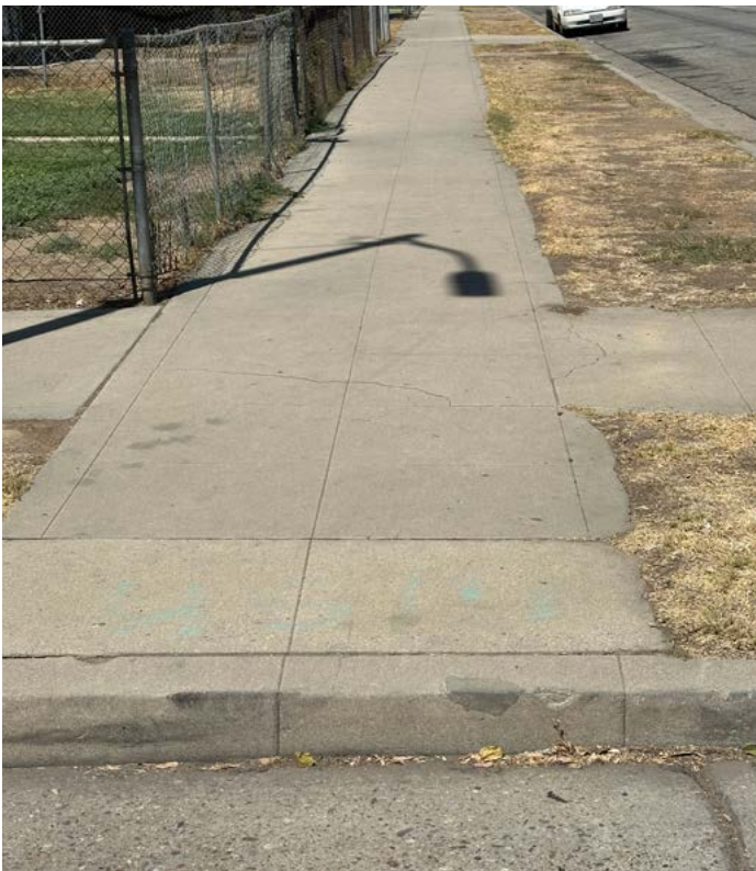
ABOVE: The Monterey Street/Alta Vista Drive intersection sidewalk has no curb ramp.
