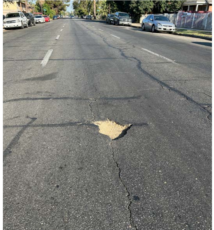
ABOVE: Monterey Street is a one-way, three-lane road that drivers use as a thoroughfare even though it is largely residential. A pothole can be seen in the road.
