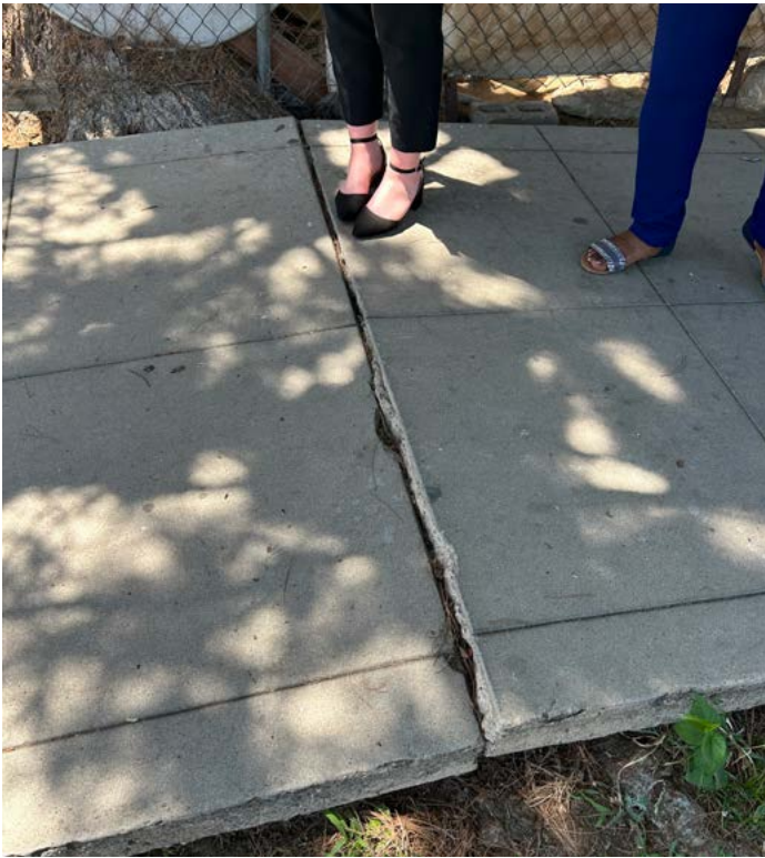
ABOVE: An uneven sidewalk due to an uprooted tree in front of a home on the south side of the Monterey Street/Haley Street intersection creates unsafe conditions by posing a tripping or fall hazard for pedestrians.
