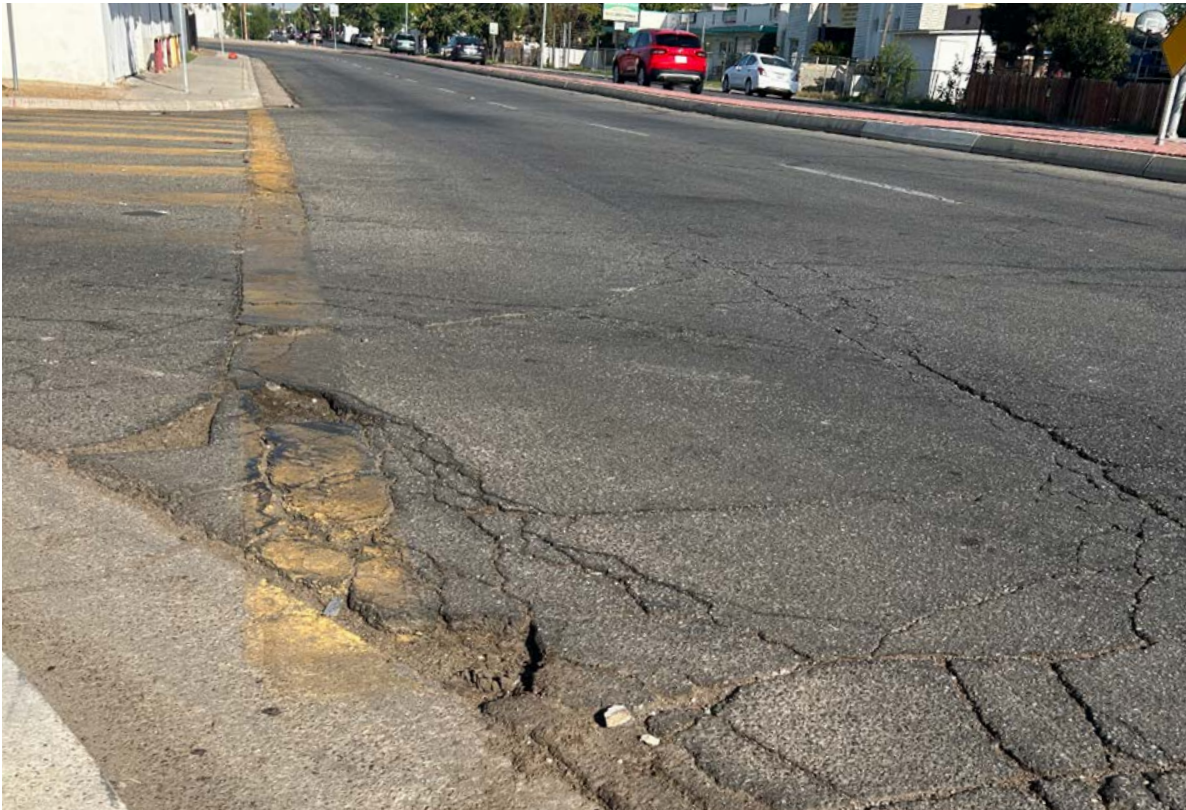
ABOVE: Potholes, like the ones located at the Williams Street/Niles Street intersection, become flooded during the rainy season. Flooding poses a hazard, decreasing visibility of potholes and cracks in roads in sidewalks that may otherwise be seen when roads are not flooded.
