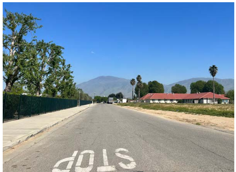
ABOVE: Grapevine Drive is missing sidewalks and lane markings.
