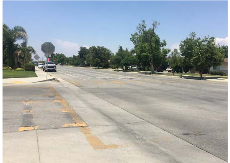
ABOVE: The high-visibility crosswalks at Grapevine Drive/Campus Drive are almost completely faded.
