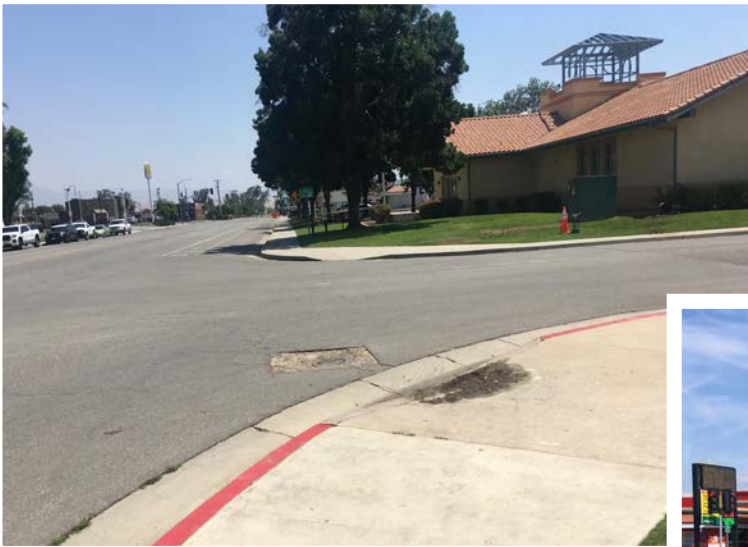
ABOVE: The west side of the 4th Street/Campus Drive intersection lacks a marked crosswalk, truncated domes on the curb ramp, and a stop sign. The buildup of debris in the curb ramp could also become a drainage problem.
