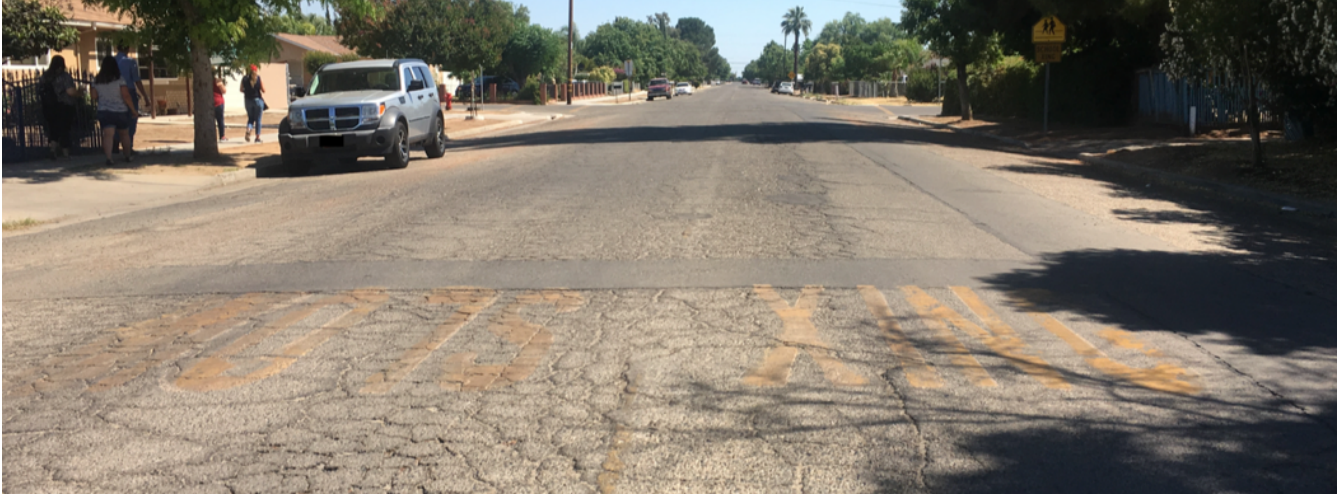
Faded and difficult to see pavement markings.
