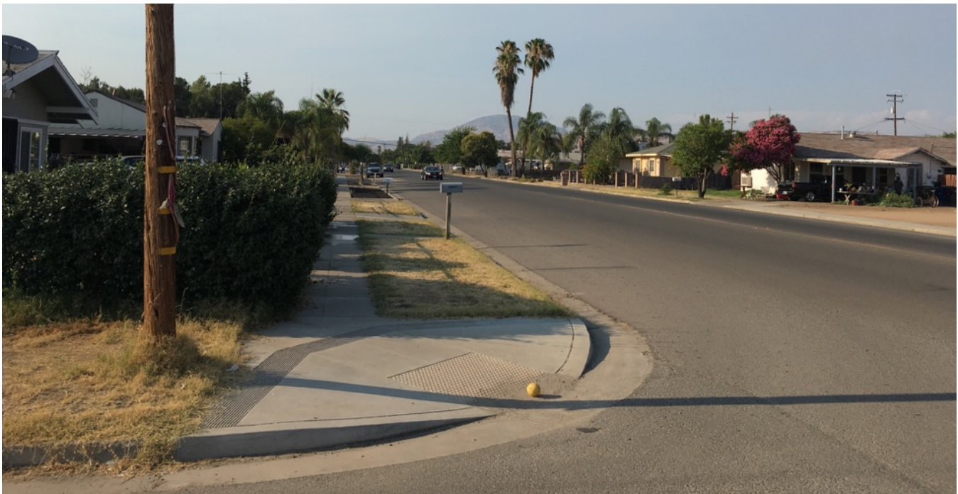
Very narrow sidewalk with overgrown vegetation beginning to obstruct the sidewalk. Silt and debris in the curb ramp indicate that there are drainage issues in the rainy season.
